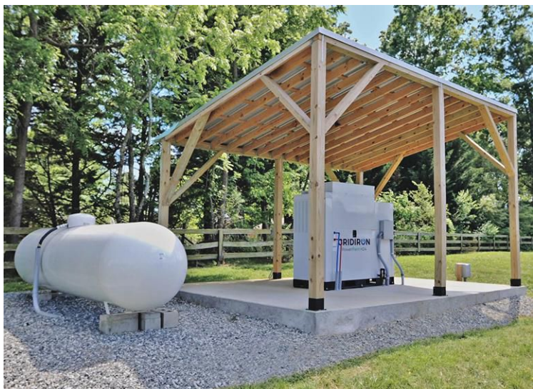
A propane tank provides fuel for a CHP system.
