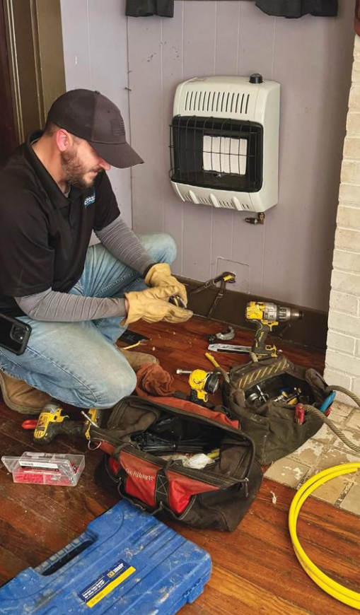
Chris Ball of Mooresville Oil & Propane restores home comfort to those affected by Hurricane Helene.
